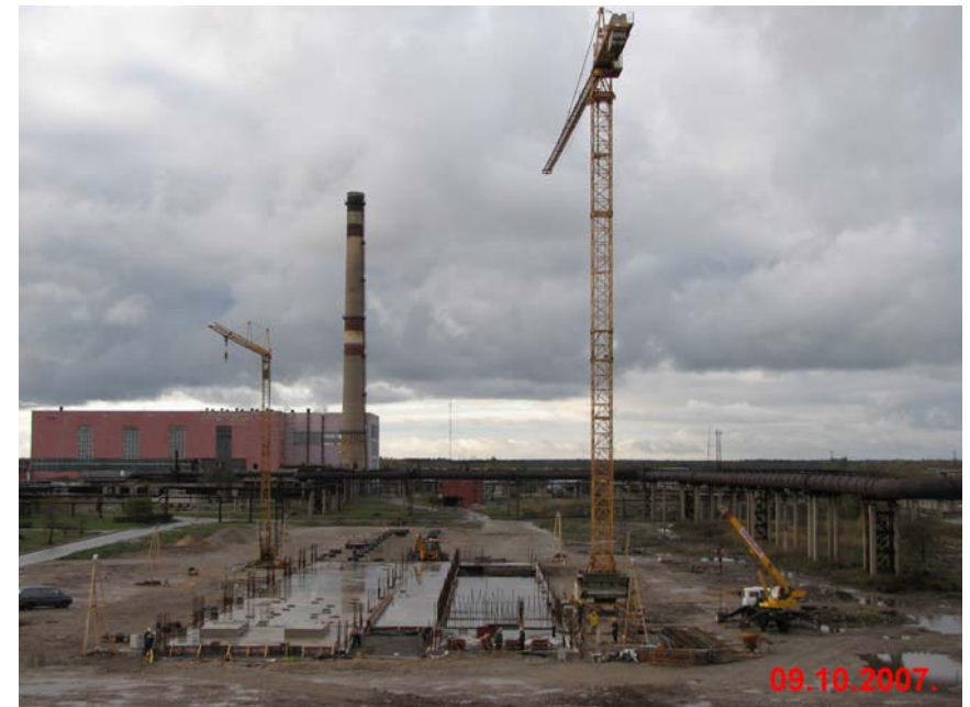
Foundation of UTT-3000 on Viru Keemia Group Galoter Project Site in Kohtla Yarve, Estonia, made under ATOMENERGOPROEKT's design, 9 th Oct, 2007
