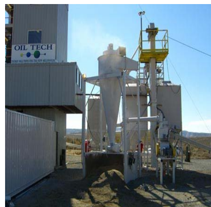
Figure 9: Dust Collector & Rock Processing Equipment
