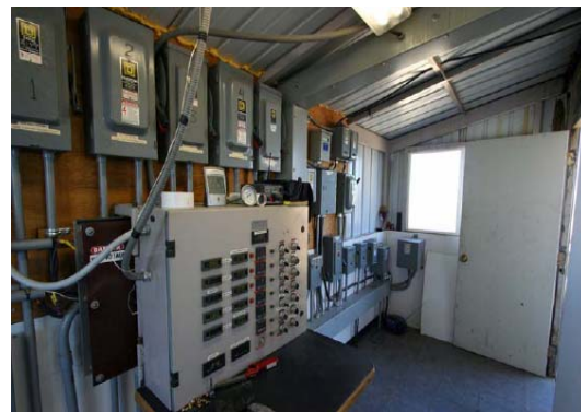
Figure 8: Retort Control Room.
