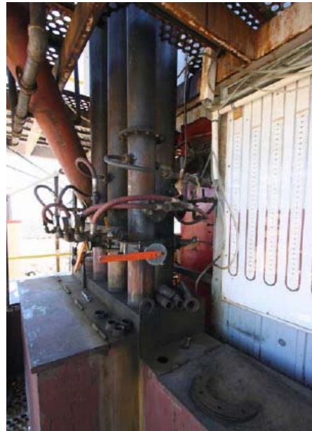
Figure 7: Condensing System Control.
